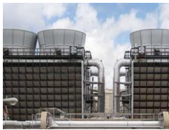
Cooling Tower Treatment Chemicals
